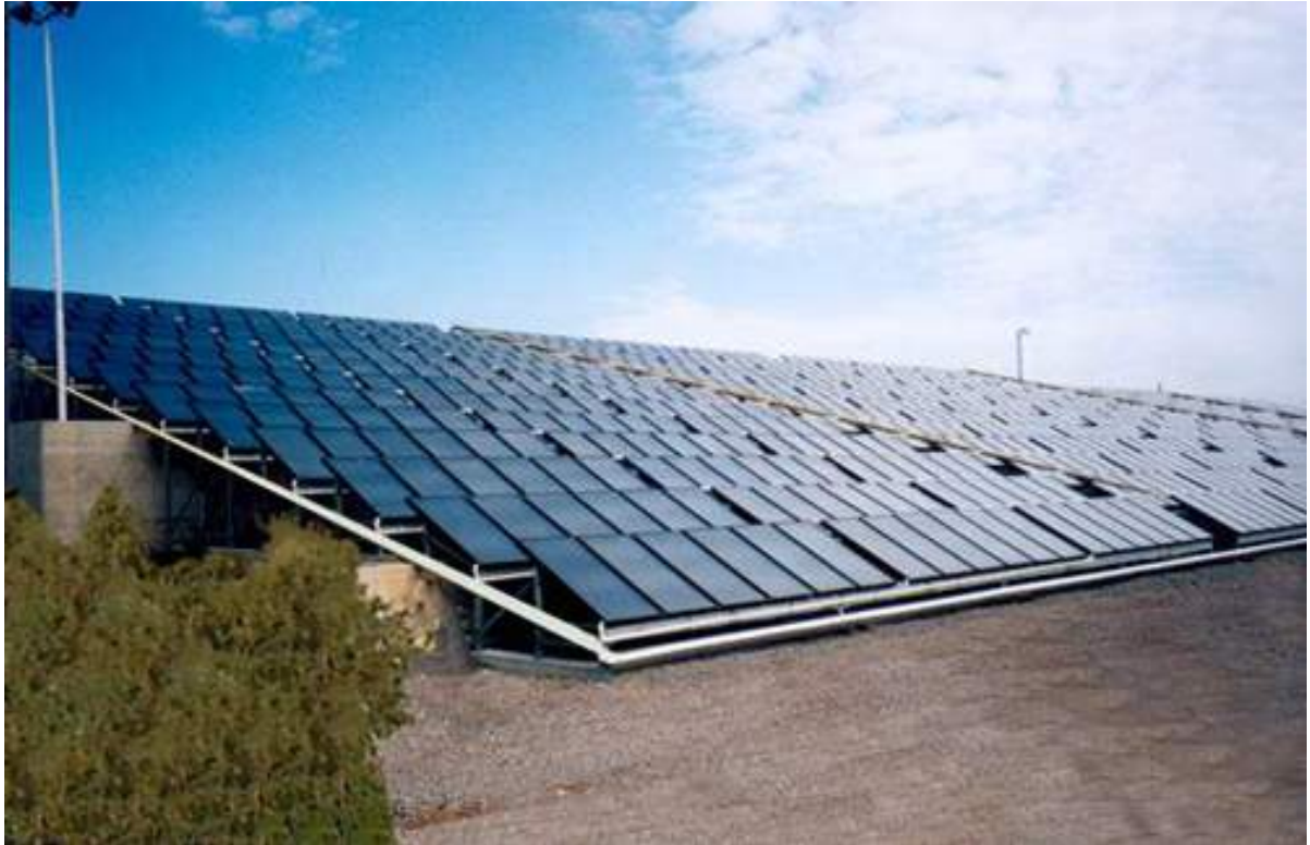
Figure 1: Solar station "PHOTONIO", Sarantis S.A.
