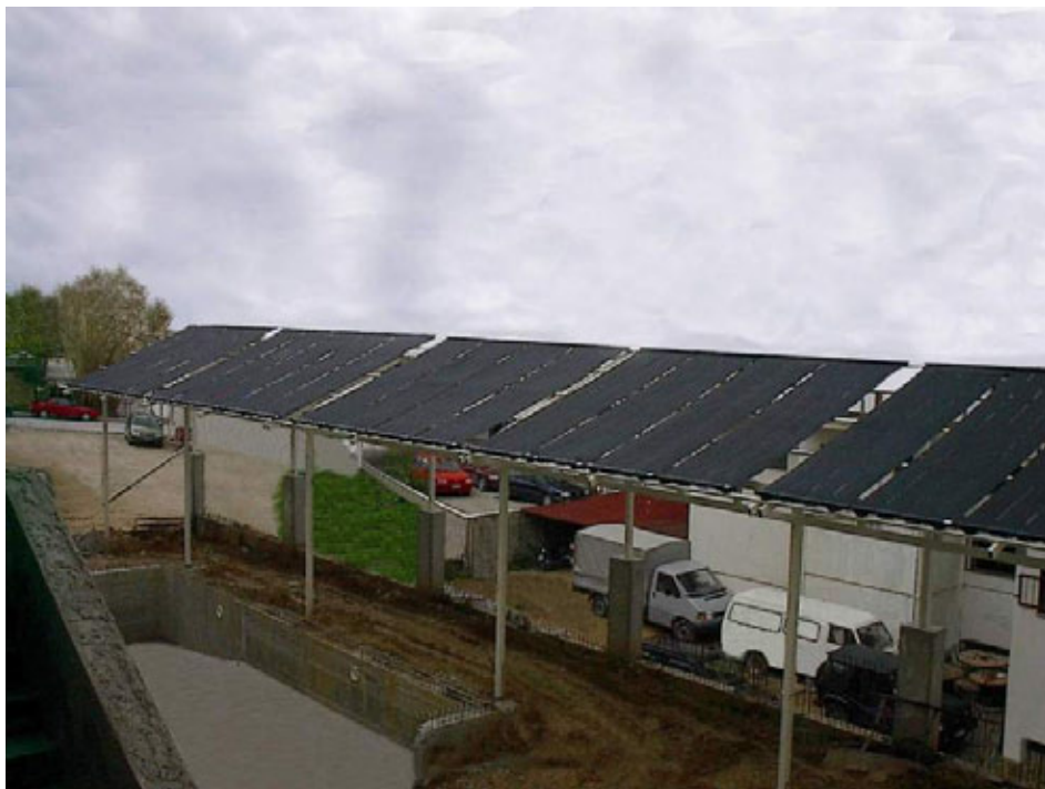
Picture 6: Solar polypropylene collectors for swimming pool heating
