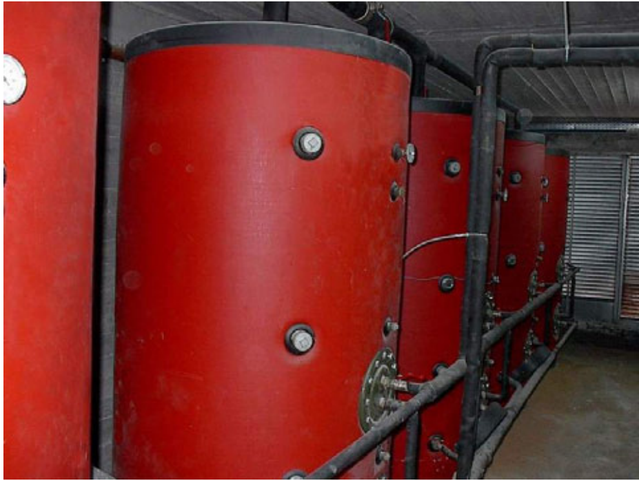
Picture 5: Plant room “LENTZAKIS A.E.” hotel
