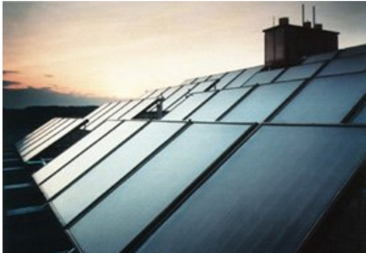
Picture 2: View of the installed solar collects of “LENTZAKIS A.E.” hotel
