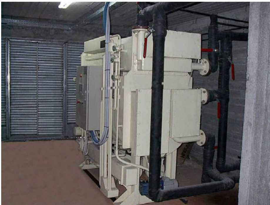
Picture 4 : Absorption chiller
