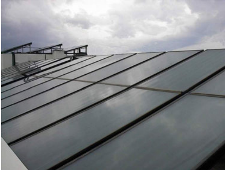
Picture 1 : The solar collectors (448 m 2 ) of “LENTZAKIS A.E.” hotel, located on the roof of the hotel.
