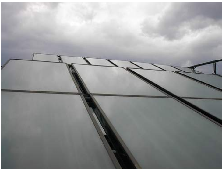
Picture 3: Different view of the installation, “LENTZAKIS A.E.” hotel
