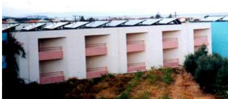
Picture 2: View of the installed solar collects of Rethimno Village hotel
