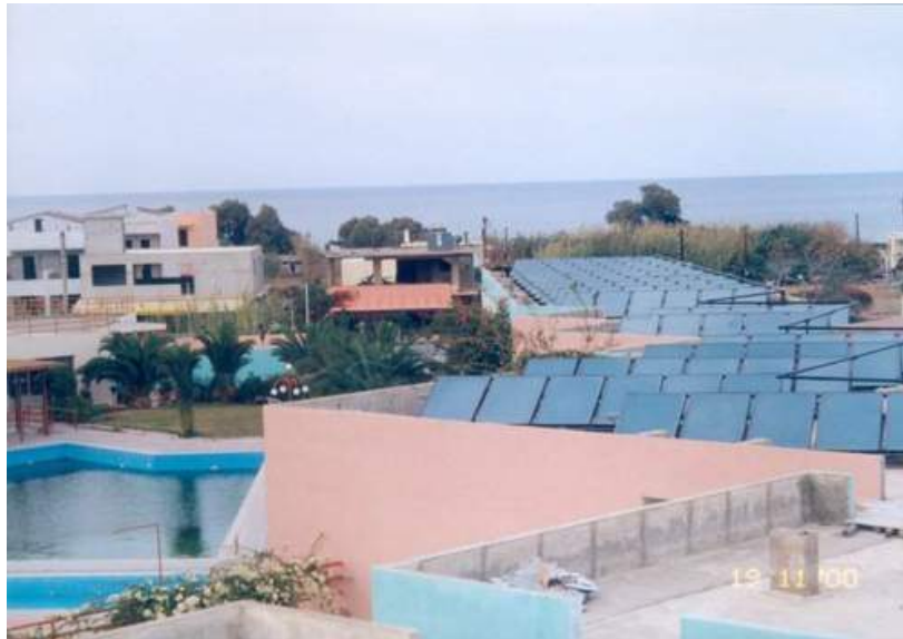
Picture 1 : The solar collectors (647 m 2 ) of Rethimno Village hotel, located on the roof of the hotel.
